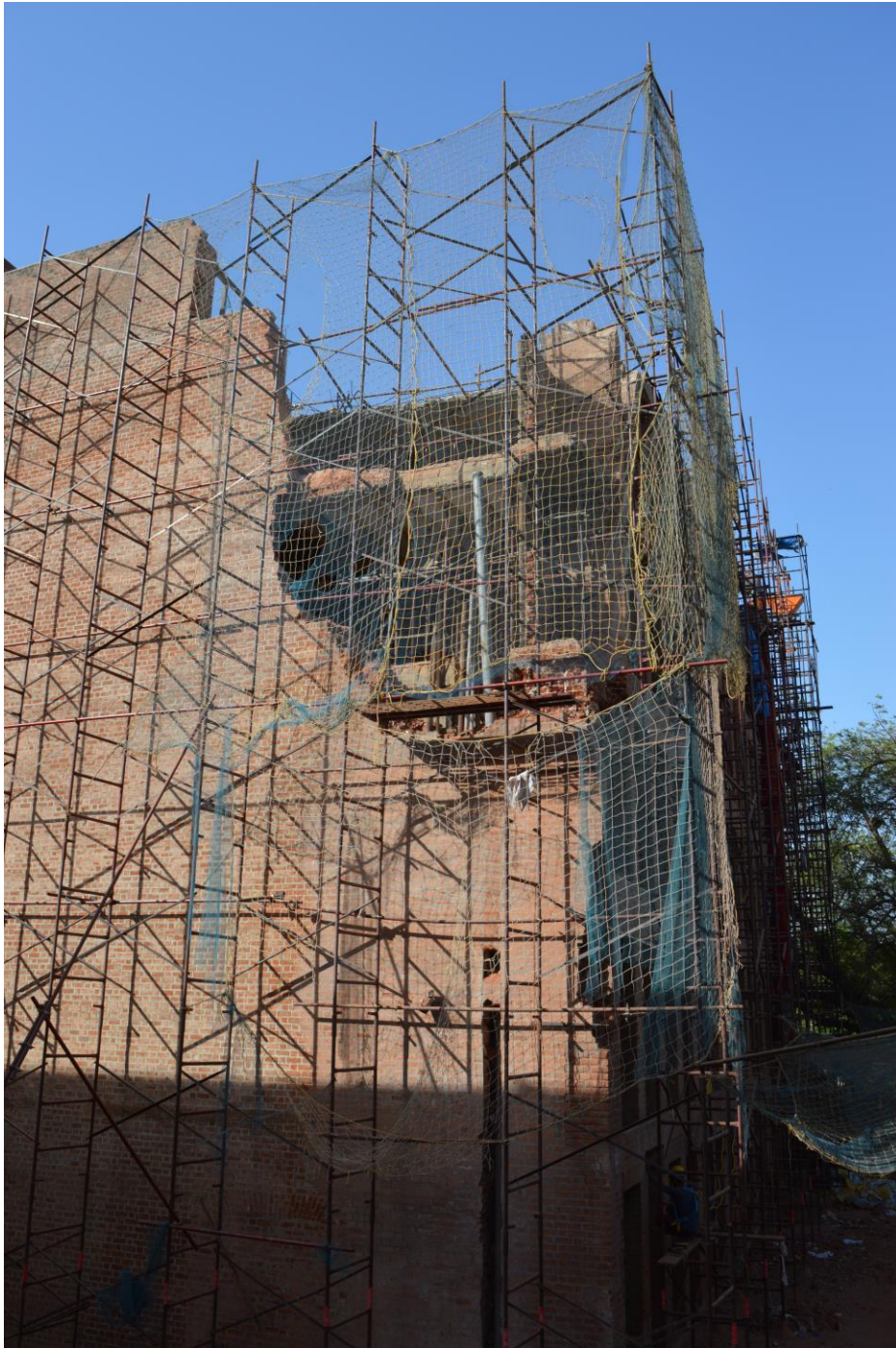
The south face of the VSL during restoration. Many of the bricks were replaced. Can we identify it as a Louis Kahn building when the restoration is complete?
